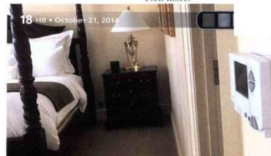
A guestroom at the J.W. Marriott Miami with a recently installed EcoSmart thermostat
